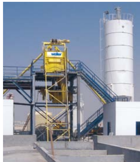
Automated concrete batching plant
